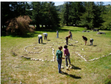
Construction of a student-designed labyrinth inspired by the natural form of an oak tree
